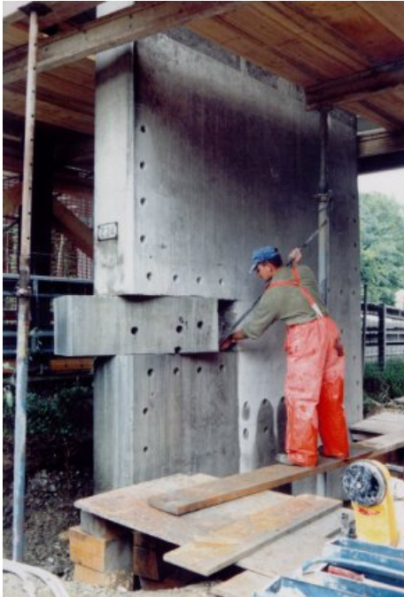
Figure 3.29: Bridge Z24: damage of the inner right pier
