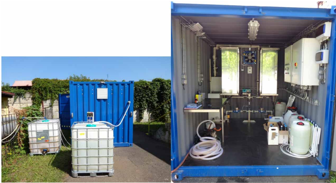
Figure 2 | The appearance of the pilot scale unit, operated on an industrial site, in a container: left, outside view; right, interior of container with two visible reactors.
