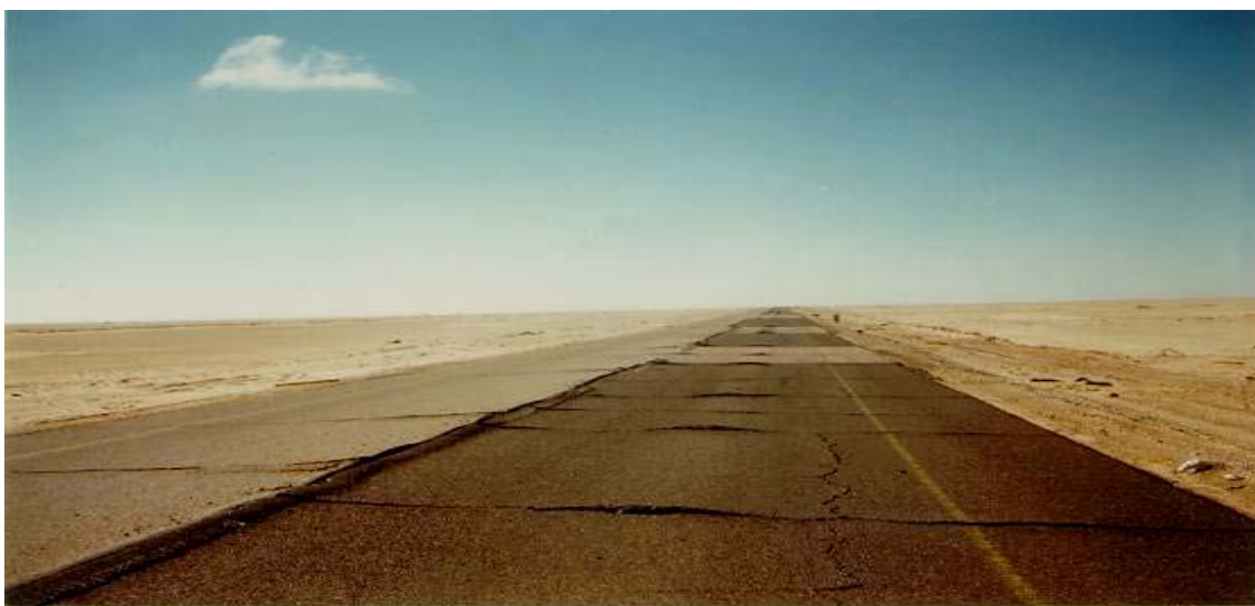
Figure 3.2 Longitudinal and transverse cracking appears again after repair work
