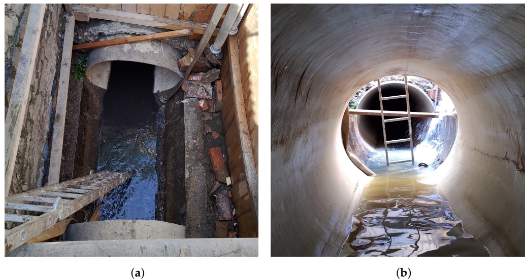
Figure 2. Example of in situ retrofitting action from Brno Lužánky park: (a) Image of the dugged starting shaft; (b) Image from inside the newly cured pipe in the old, damaged sewage pipe. Images taken by Prof. Luboš Pazdera.
