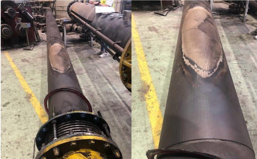
Fig. 47 Damaged pulverised coal channel - Eroded area
