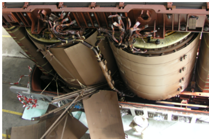
Fig. 1.2: Solid insulation of power transformer 2AT3 in ETE used in Temelin
