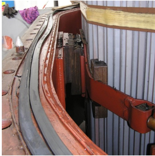
Fig. 3.2: Dismantled transformer with rubber gasket inside the gap
