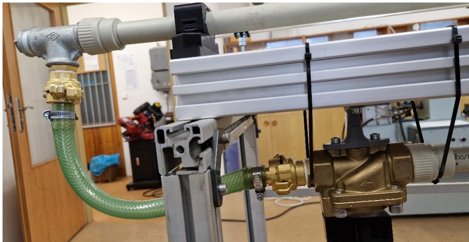
Fig. 55 One end of the connected air distribution.
