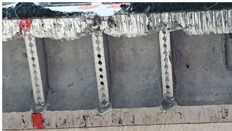
Figure 2.3 Destructive method of investigation clogged channels.
